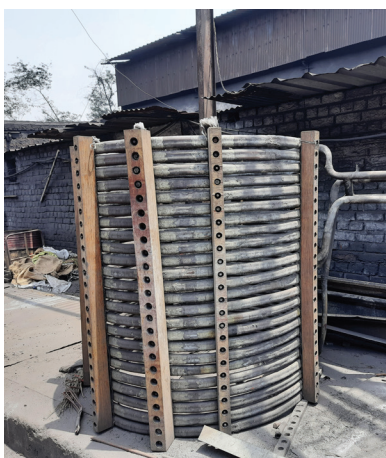
Figure 37: Copper coil in induction furnace
