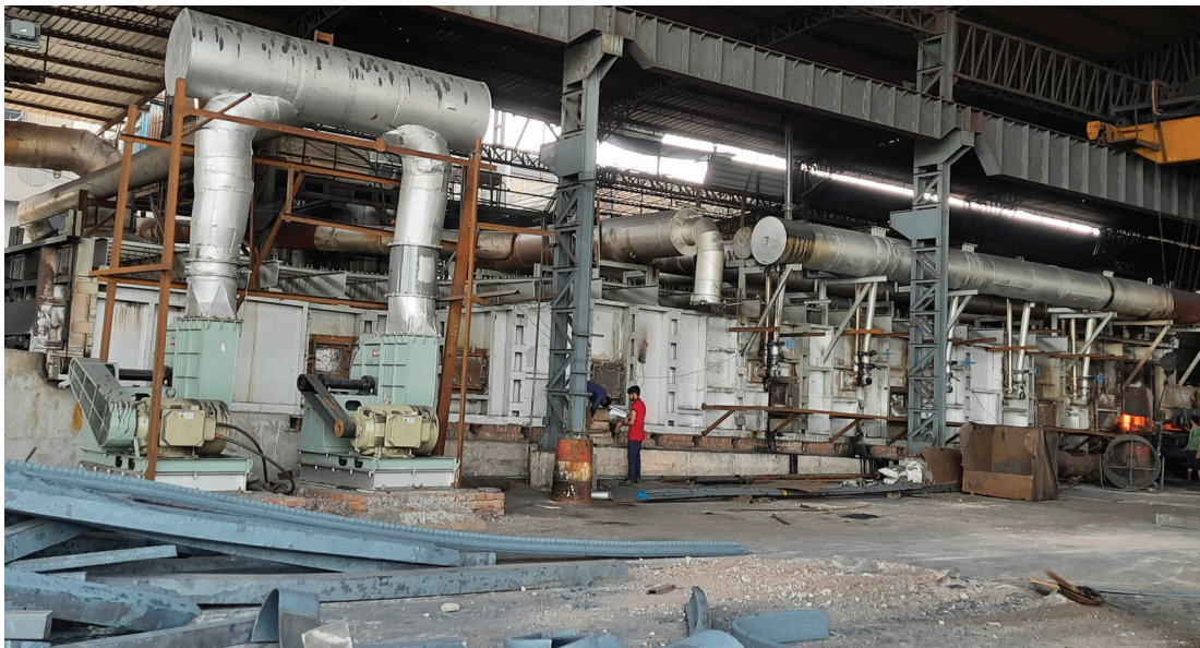
Figure 45: View of re-heating furnace
