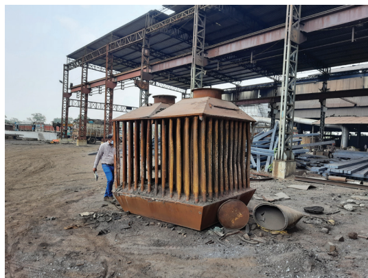
Figure 47: View of recuperator
